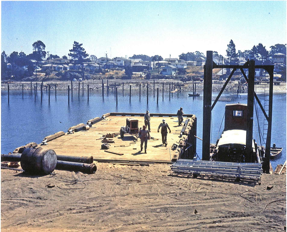
Figure 53. The Public Pier complete. Anchor piles in place for floatation units in the distance.
