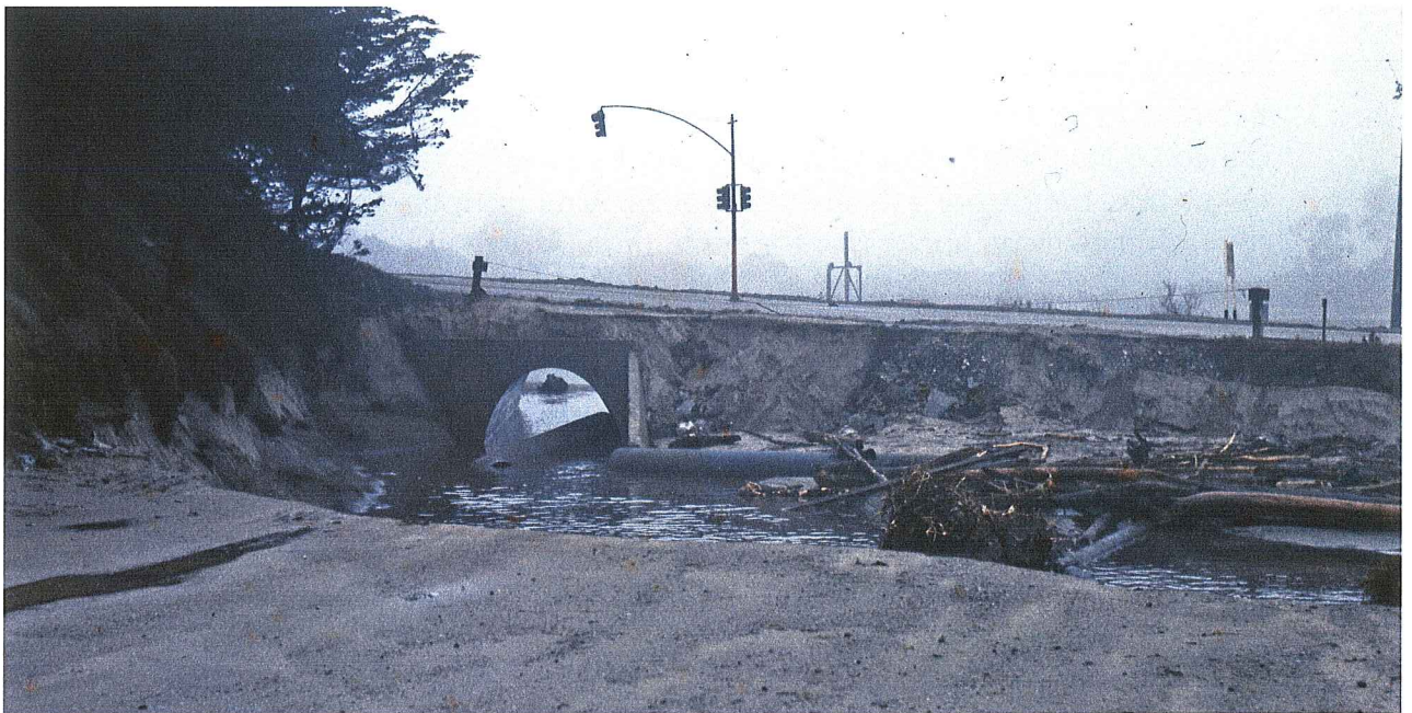
Figure 2. East Cliff Drive before the Harbor. Bridge is a Corrugated Metal Arch attached to a Concrete slab on footings, with headwalls.
