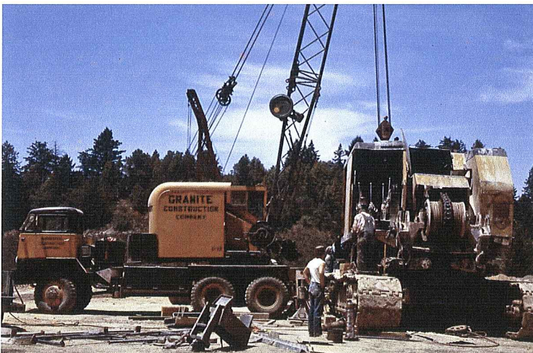
Figure 8. Assembling the crane. It takes a small one to lift the parts onto the big one.
