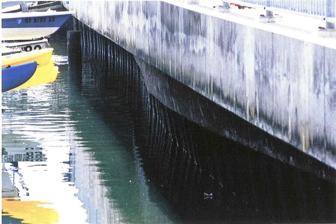
Figure 49 a. Damaged bulkhead with the concrete cap built over it.
