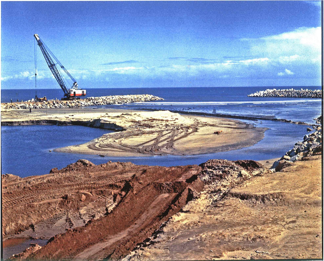
Fig. No. 7. Inner view. Working on the east jetty. West jetty on the right is complete.
