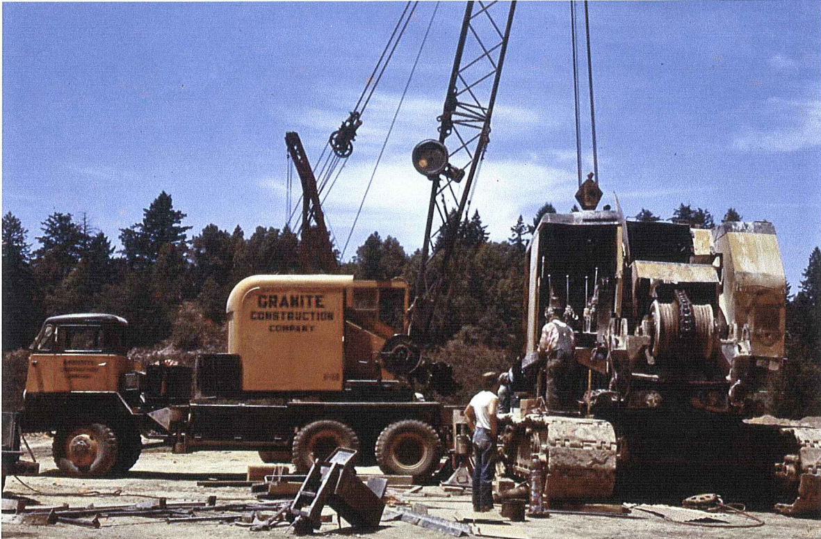
Figure 8. Assembling the crane. It takes a small one to lift the parts onto the big one.
