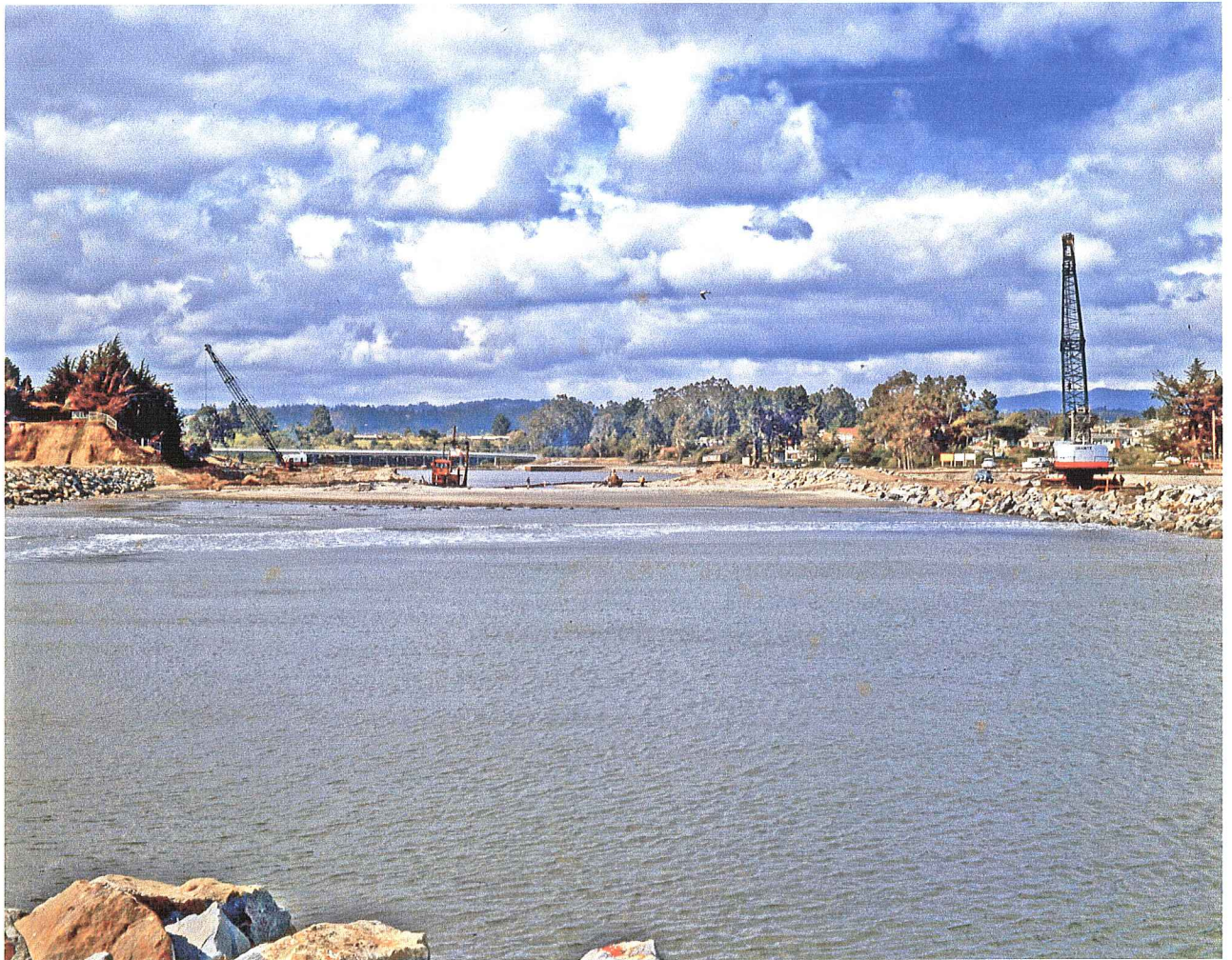
Fig No. 9. Digging through the beach. Working in the breakers to open the harbor. (Taken from the end of the completed west jetty, facing north. (Bx7-SL10-img 125)
