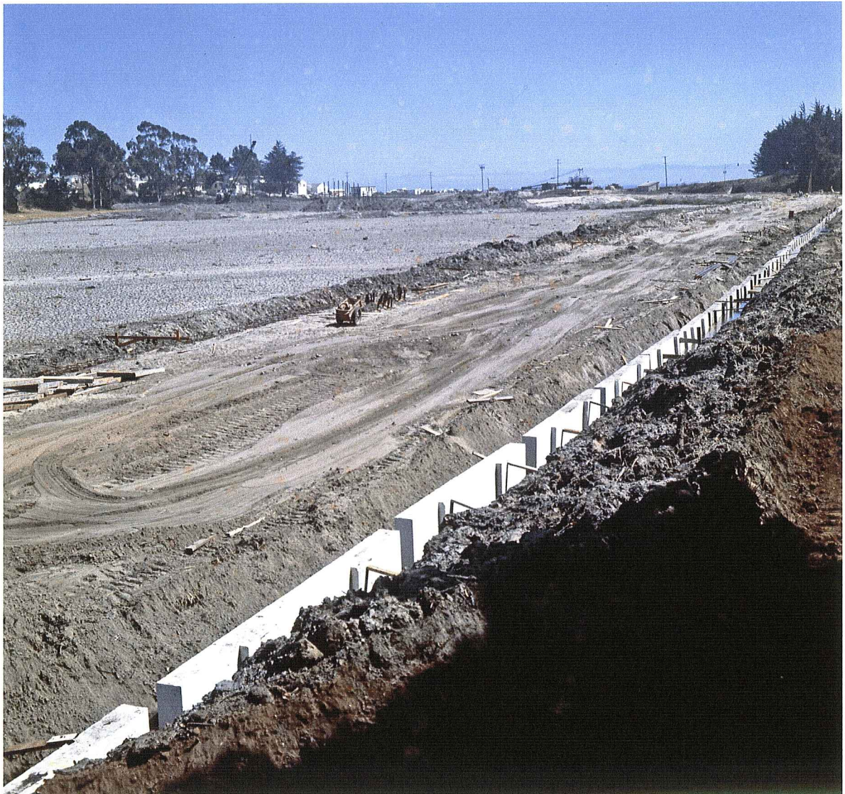
Figure 48. West Bulkhead. Steel sheet piling in place. Before the damage. Facing south.
