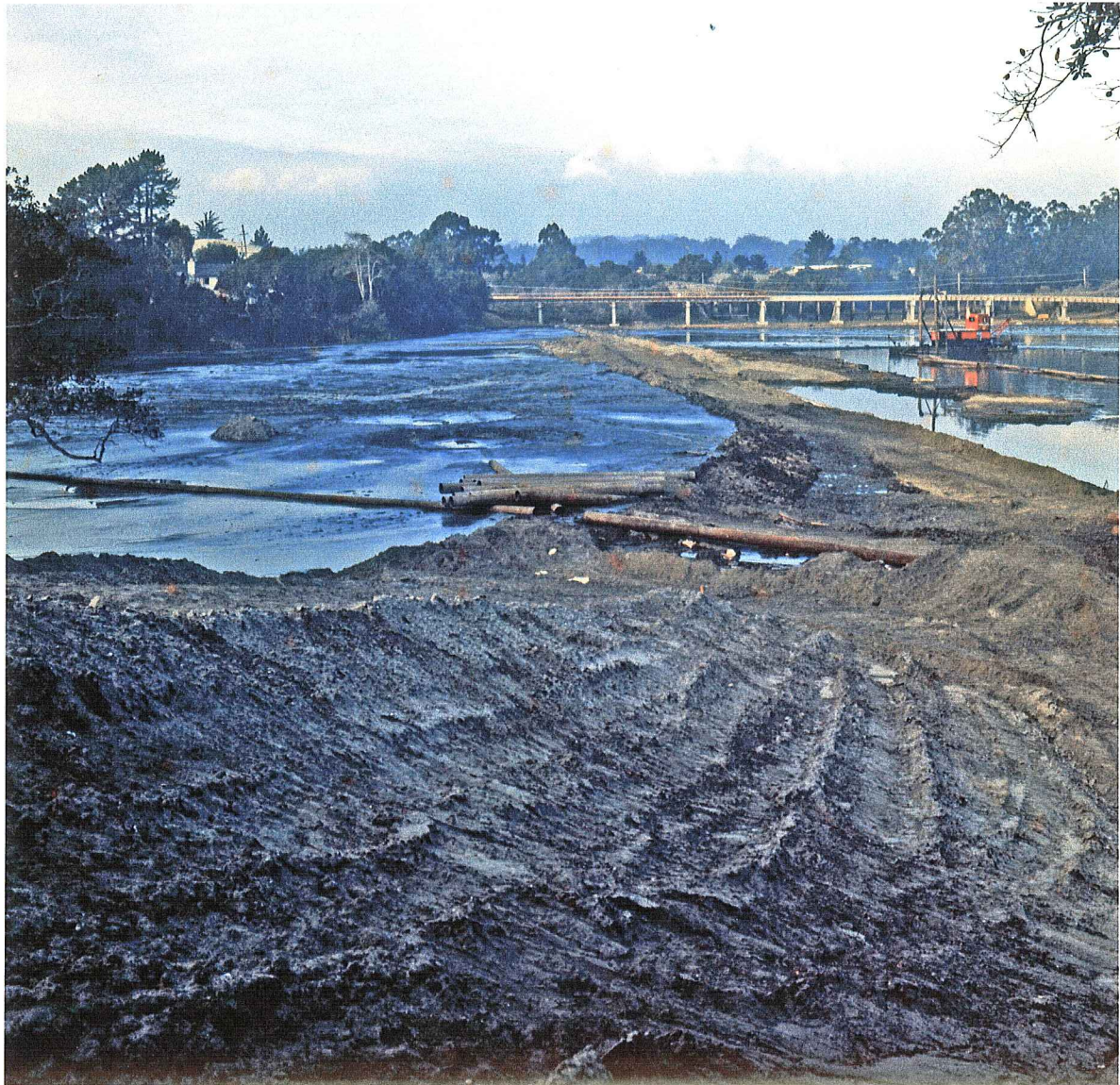
Fig. No. 2. Filling west parking lot with pumped in material. Shellmaker's dredge working in the distance.
