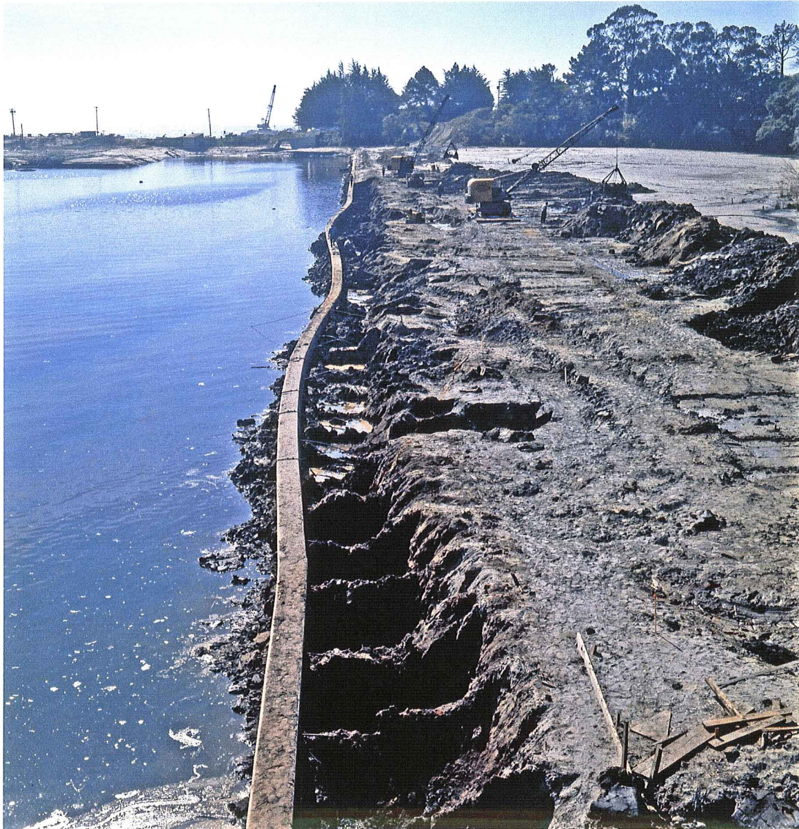
Fig.49. The damaged bulkhead wall.
