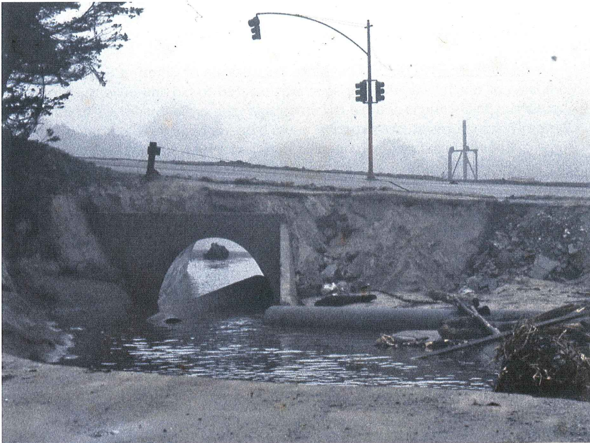
Figure 3. Blown up picture of corrugated metal arch culvert, which is the Woods Lagoon outlet. A log is floating in the culvert.
