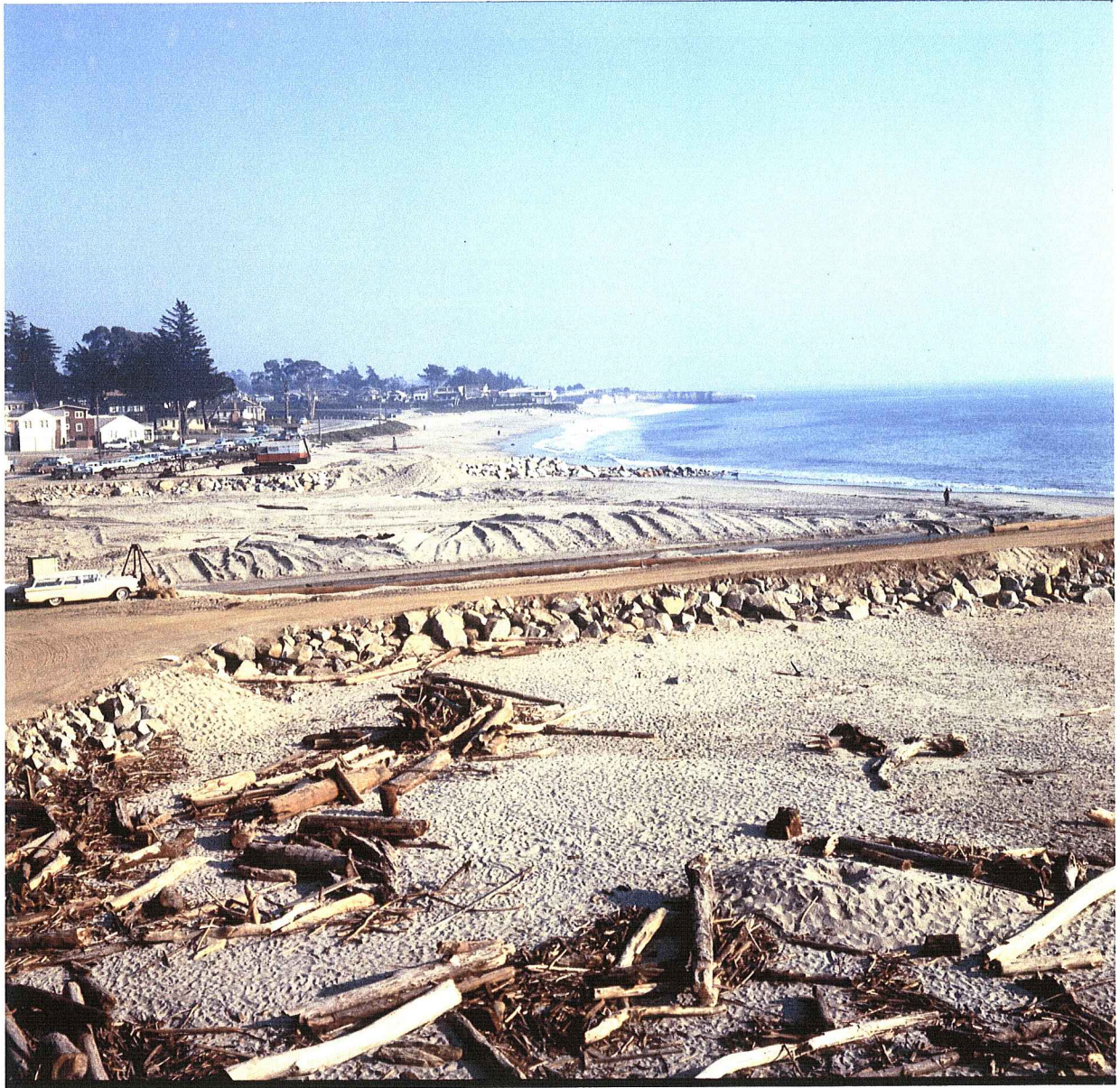
Fig. No. 6. West jetty is complete. Working on east jetty in the distance.
