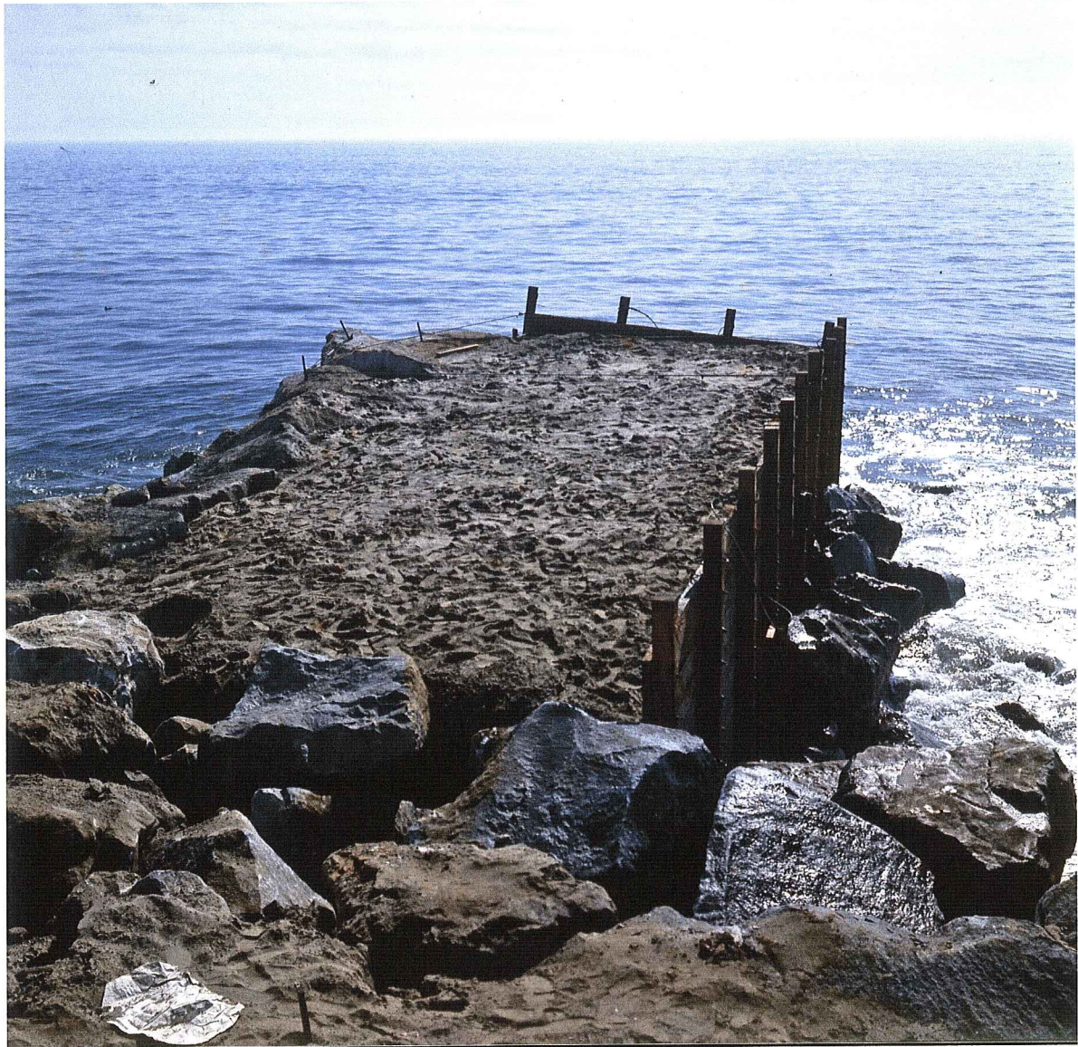
Fig. No. 1. Section at end of spine, on west jetty filled with fresh grout.
