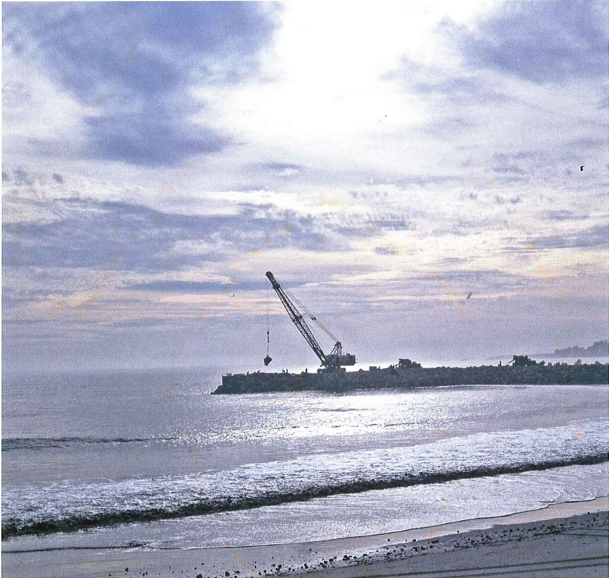
Figure 61. Working late to finish a section of the concrete spine before the storm.
