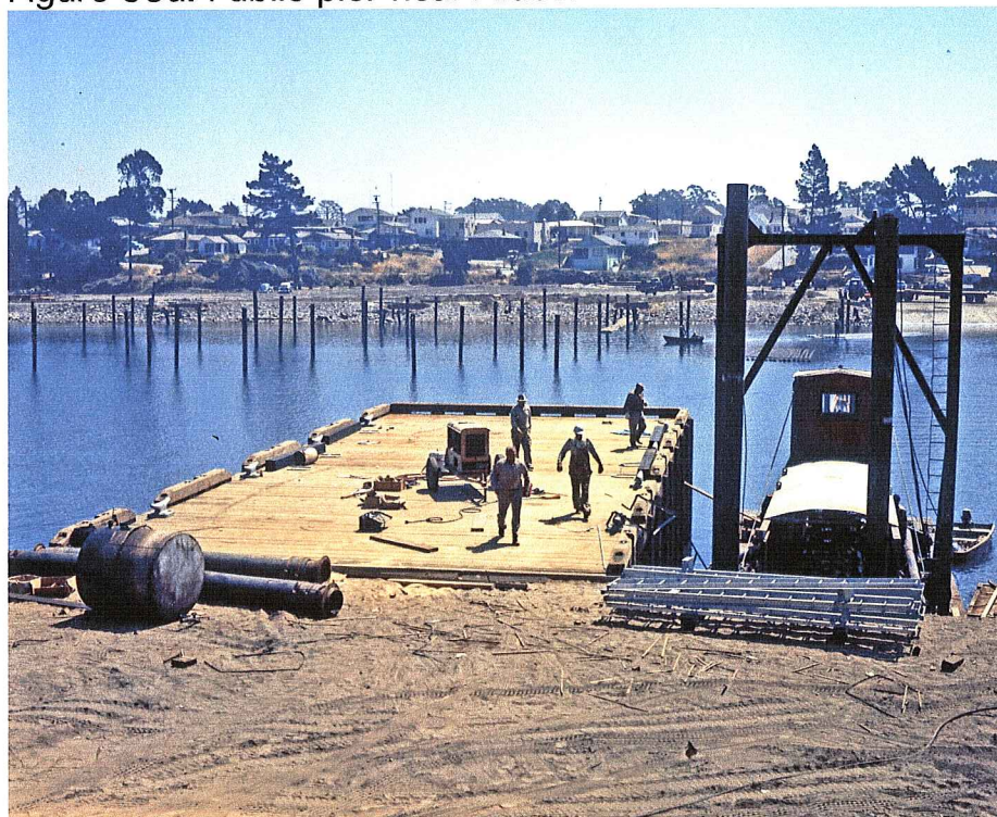
Figure 53. The Public Pier under construction. Anchor piles in place for floatation units, in the distance. Aldo's is now to the right of this pier.
