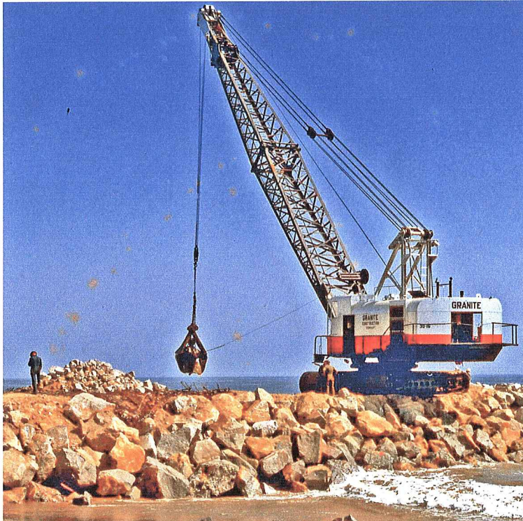
Figure 38. Crane working on the East Jetty. Notice the sand, before the harbor mouth was opened.
