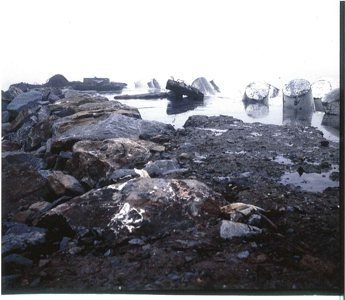
Fig. No. 3. Top of the west jetty after the storm.
