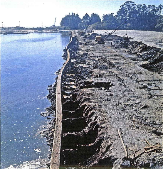
Figure 49. Exposed damaged bulkhead before repair. Facing South.
